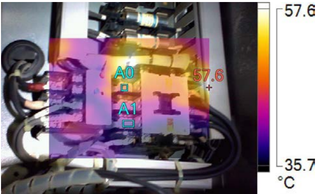
IR005210.IS2-Air Cond SW pump
