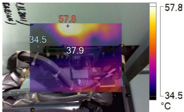
IR005171.IS2-Scrubber Pump 12/3/2016 11:17:48 AM
