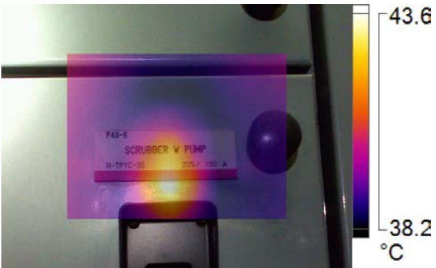
IR005165.IS2-Scrubber Pump 12/3/2016 11:13:59 AM
