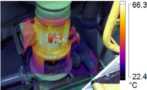
IR005225.IS2-Air Cond SW pump
