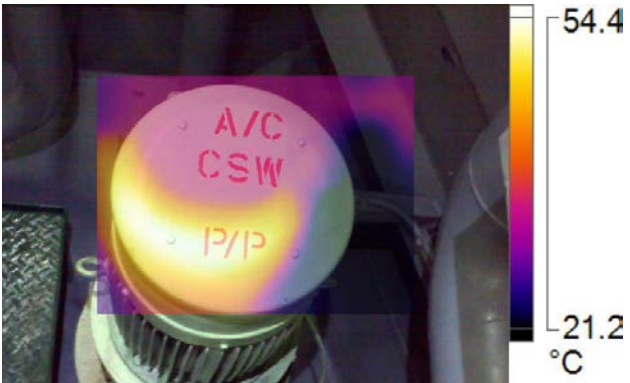
IR005222.IS2-Air Cond SW pump
