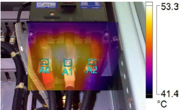
IR005167.IS2-Scrubber Pump 12/3/2016 11:16:04 AM
