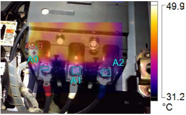
IR005209.IS2-Air Cond SW pump
