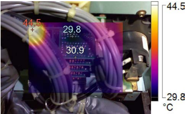
IR005122.IS2-No2 Jacket water pump 12/3/2016 8:52:05 AM
