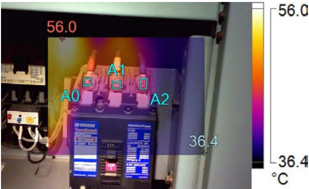
IR005201.IS2-No2 SW Serv pump 12/3/2016 1:22:22 PM
