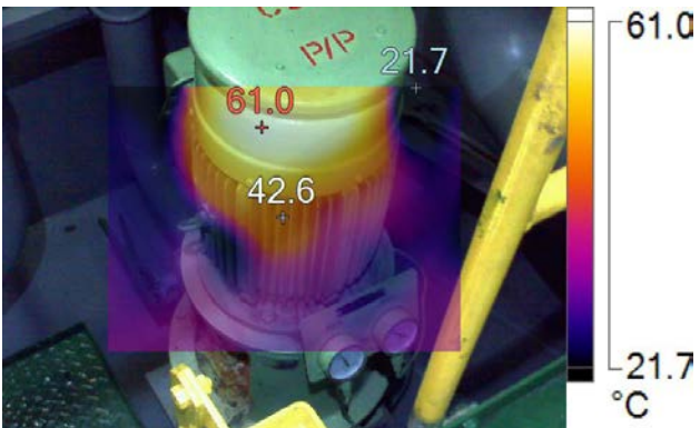
IR005223.IS2-Air Cond SW pump
