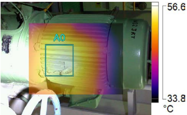
IR005125.IS2-No2 Jacket water pump 12/3/2016 8:53:38 AM
