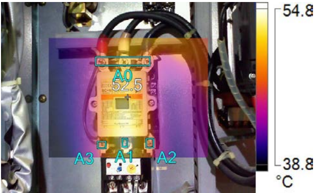
IR005168.IS2-Scrubber Pump 12/3/2016 11:16:39 AM
