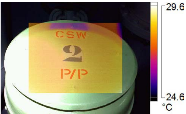
IR005141.IS2-No2 CSW pump 12/3/2016 9:22:14 AM
