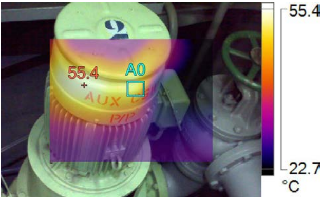
IR005213.IS2-Air Cond SW pump
