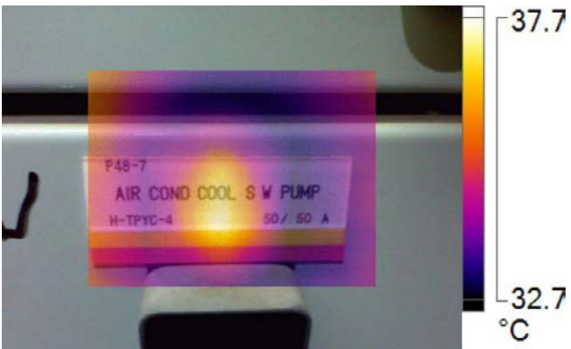
IR005207.IS2-Air Cond SW pump 12/3/2016 1:27:25 PM
