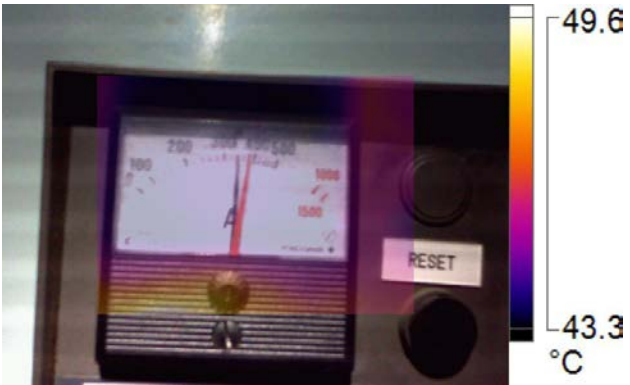
IR005934.IS2-No2 Ballast pump panel 12/5/2016 8:22:31 PM
