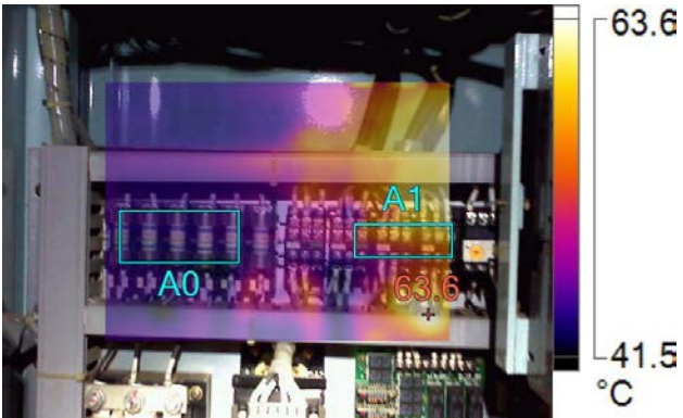
IR005947.IS2-No2 Ballast pump panel 12/5/2016 8:25:53 PM
