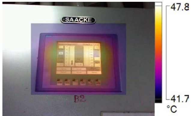
IR005864.IS2-Boilers panel 12/5/2016 5:37:00 PM
