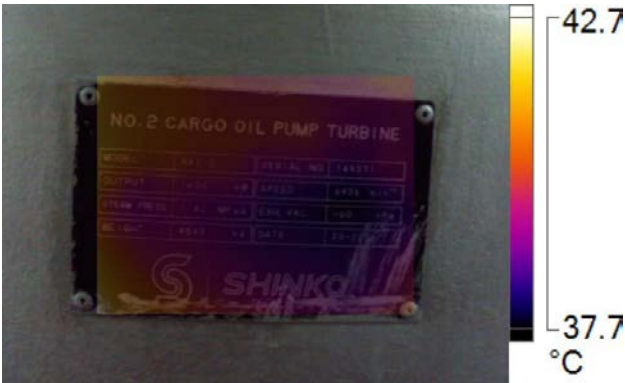
IR005799.IS2-No2 Cargo Turbine 12/5/2016 1:26:39 PM
