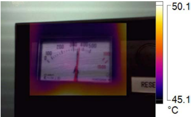
IR005908.IS2-No 1 Ballast pump panel 12/5/2016 8:12:44 PM
