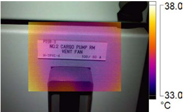
IR005969.IS2-No 2 Pump room fan 12/6/2016 9:26:58 AM
