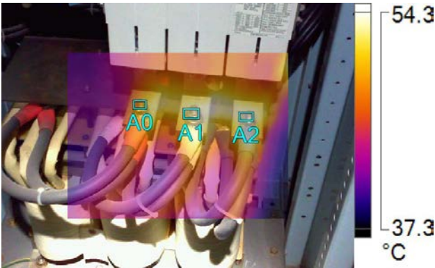
IR005940.IS2-No2 Ballast pump panel 12/5/2016 8:24:26 PM
