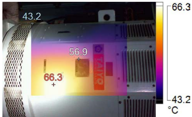
IR005927.IS2-No 1 Ballast pump 12/5/2016 8:19:11 PM
