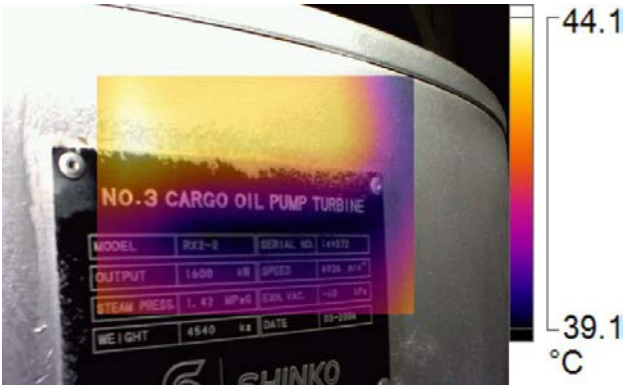
IR005813.IS2-No 3 Cargo Turbine 12/5/2016 2:43:18 PM
