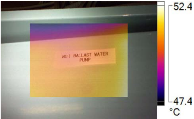
IR005907.IS2-No 1 Ballast pump panel 12/5/2016 8:12:30 PM
