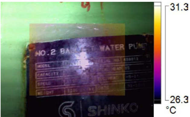
IR005903.IS2-No 2 Ballast pump
