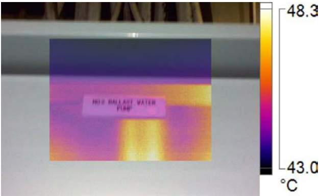
IR005933.IS2-No2 Ballast pump panel 12/5/2016 8:22:06 PM
