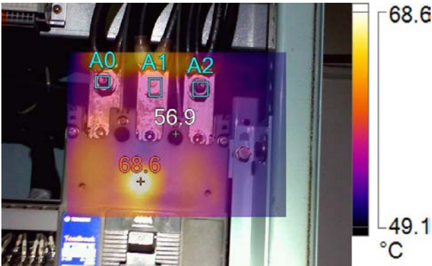
IR005923.IS2-No 1 Ballast pump panel 12/5/2016 8:17:39 PM
