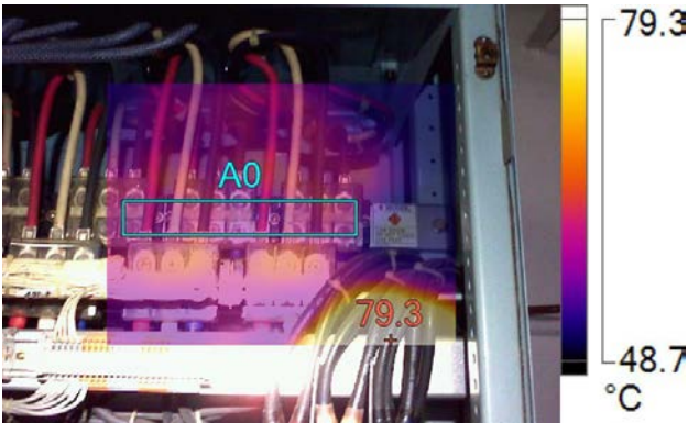
IR005922.IS2-No 1 Ballast pump panel 12/5/2016 8:17:03 PM
