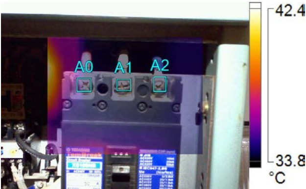
IR005965.IS2-No1 Pump room fan 12/6/2016 9:26:00 AM
