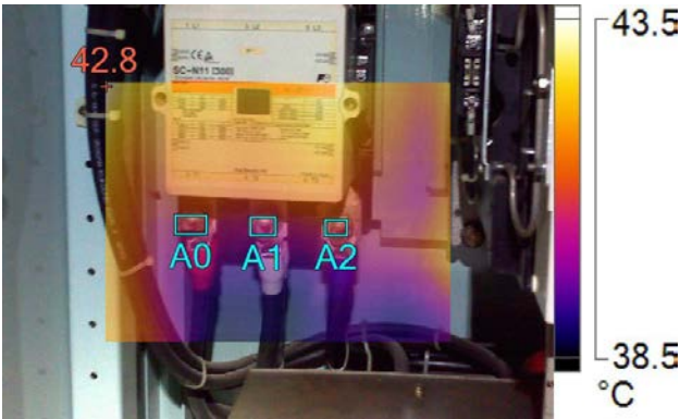
IR005943.IS2-No2 Ballast pump panel 12/5/2016 8:24:58 PM
