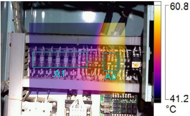
IR005945.IS2-No2 Ballast pump panel 12/5/2016 8:25:24 PM
