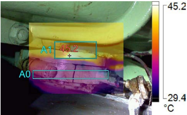
IR005809.IS2-No2 Cargo Pump 12/5/2016 2:04:51 PM
