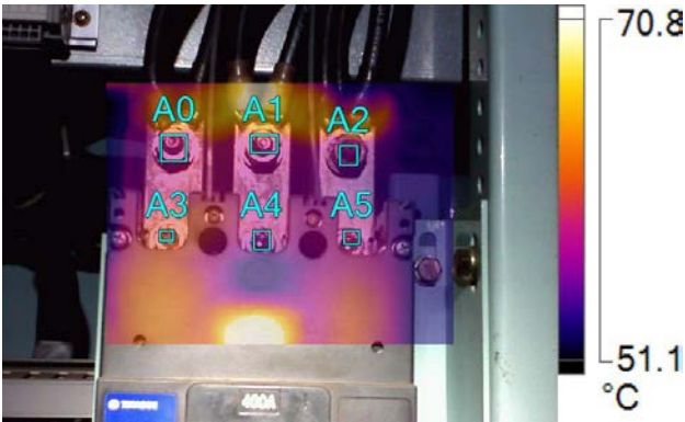
IR005924.IS2-No 1 Ballast pump panel 12/5/2016 8:17:48 PM
