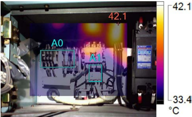
IR005967.IS2-No1 Pump room fan 12/6/2016 9:26:31 AM
