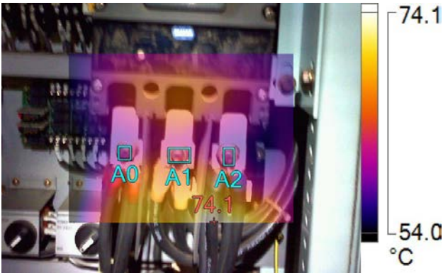
IR005911.IS2-No 1 Ballast pump panel 12/5/2016 8:13:46 PM
