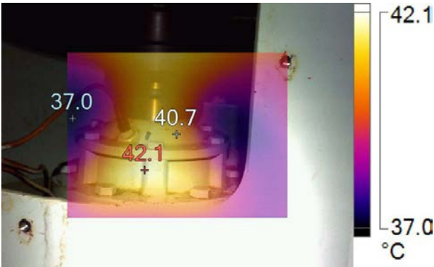
IR005958.IS2-No2 Ballast pump 12/5/2016 8:29:56 PM
